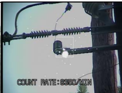
The exact corona arcing location
