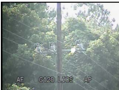
Arcing corona seen hundreds of feet away on hazy day.
