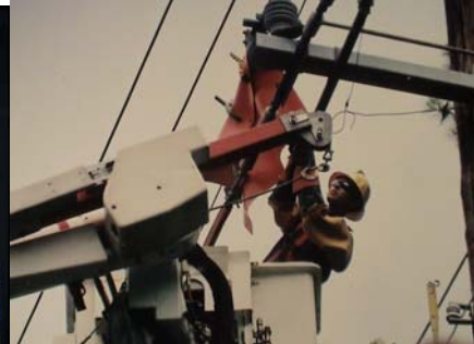
Lineman from EMC takes down the faulty arrester
